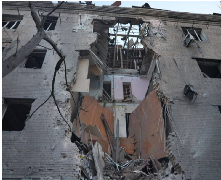
Figure 3: The stairs of a residential building destroyed by a Russian ballistic missile in the city of Zaporizhzhia, from which children and their parents are looking for a way out.
