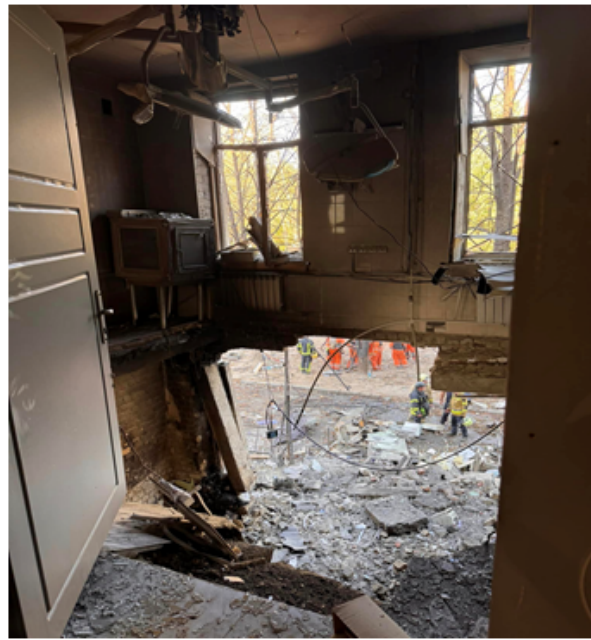
Figure 1: Configuration of the failure of the ceiling of the hospital in the city of Sumy, where she was saved some patients.
